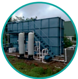
EFFLUENT TREATMENT PLANT
